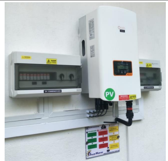
Inverter Installation Solis Three Phase 10kW
