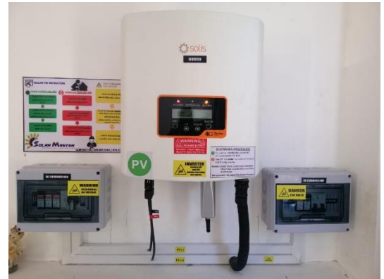
Inverter Installation Solis Single Phase 3kW
