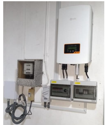
Inverter Installation Solis Single Phase 5kW
