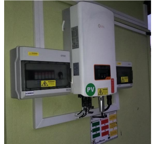
Inverter Installation Solis Single Phase 5kW
