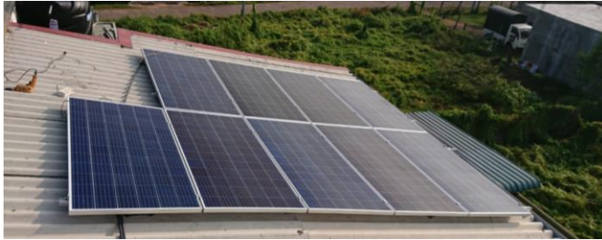
Panel Installation Amerisolar Poly Cell Module -09 Nos
