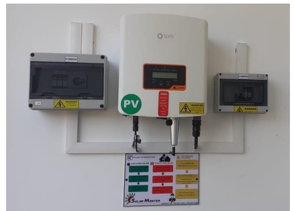
Inverter Installation Solis Single Phase 3kW
