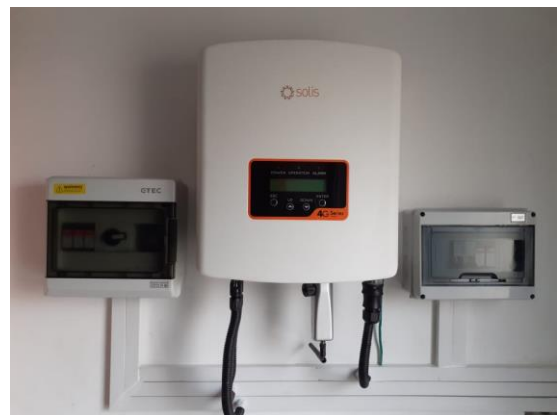
Inverter Installation Solis Single Phase 3kW
