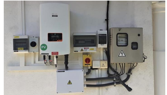
Inverter Installation Solis Three Phase 8kW
