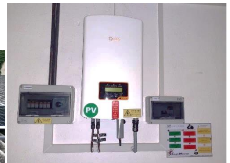
Inverter Installation Solis Single Phase 5kW
